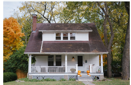
Settlement cracks in front porch... (3/3) —
