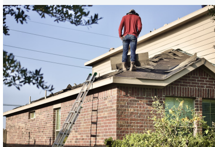
Shingle granule loss along... (2/3) — Roof,
